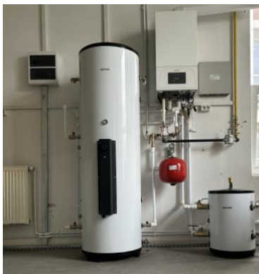
Fig. 1. The physical twin – the hybrid HVAC system
